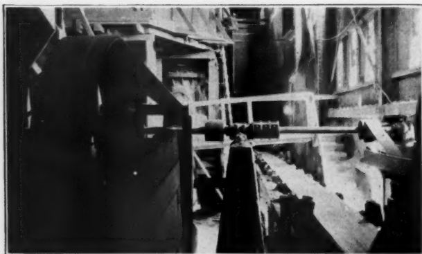
Belt Conveyor from First Scalping Screen
